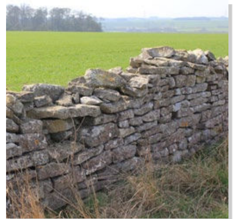
Parish boundary wall (in the ownership of the adjoining land owner to the south)
